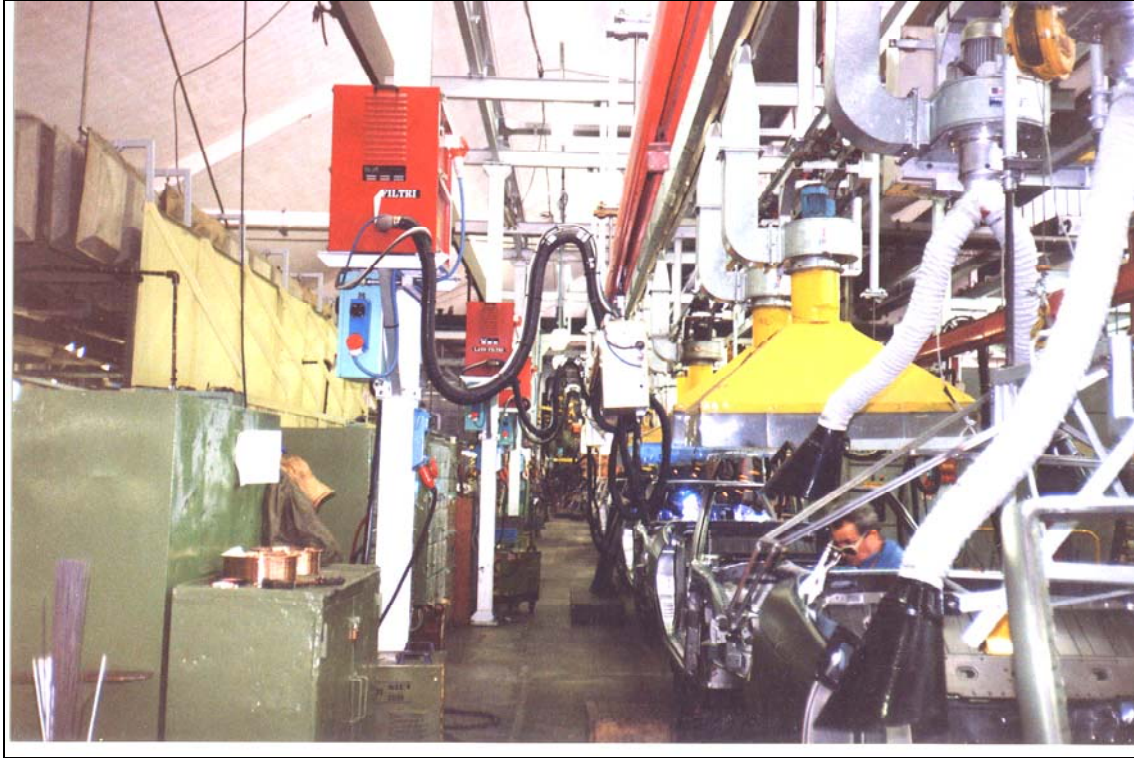
Equipping of a welding department for car bodyworks, where the equipment is fixed to a pillar and the wire feeder is installed on a monorail to follow the line skate feed to floor.
