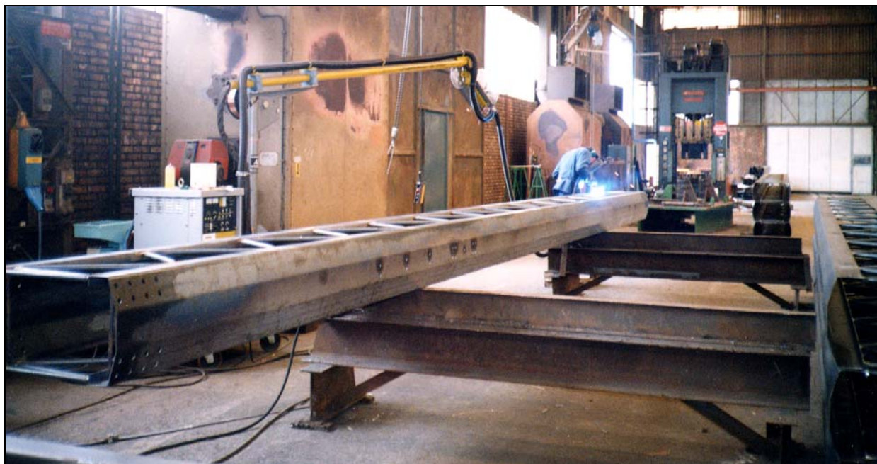
Welding of a 15 mts structure for the building industry processed in complete security either for physical hygiene or security, where wire ropes, tubes and equipments are lifted from the floor.
